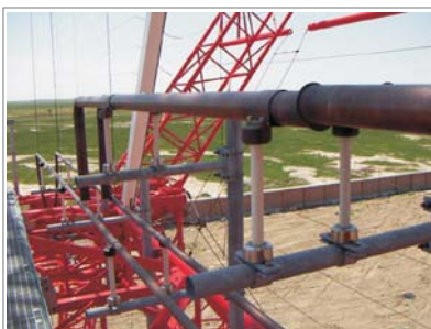
RF Feed line and catwalks
